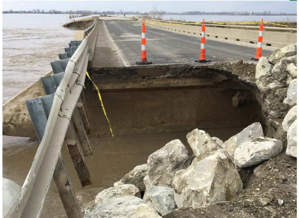
Flood damage to MO-111 following March 2019 flooding in Atchison County, MO.
