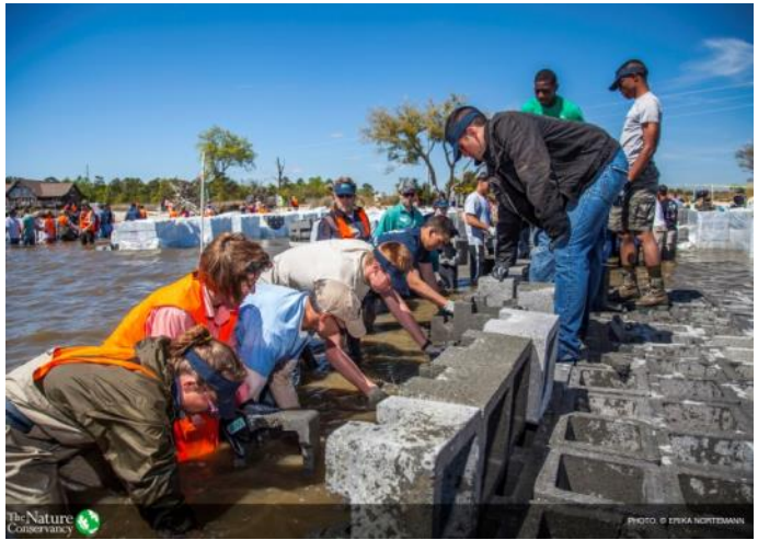
Conservancy staff, partners, and volunteers work to build the foundation for a living oyster reef shoreline in Alabama
